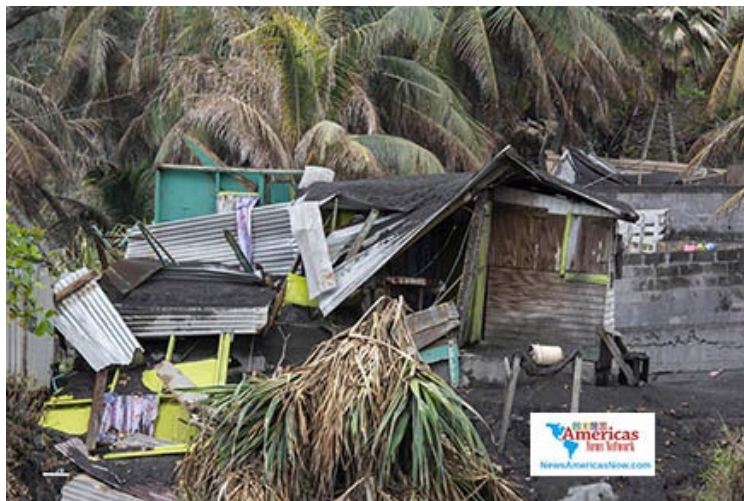
Figure 4.5 Damages to houses due to ash load. Source: NewsAmericaNow
