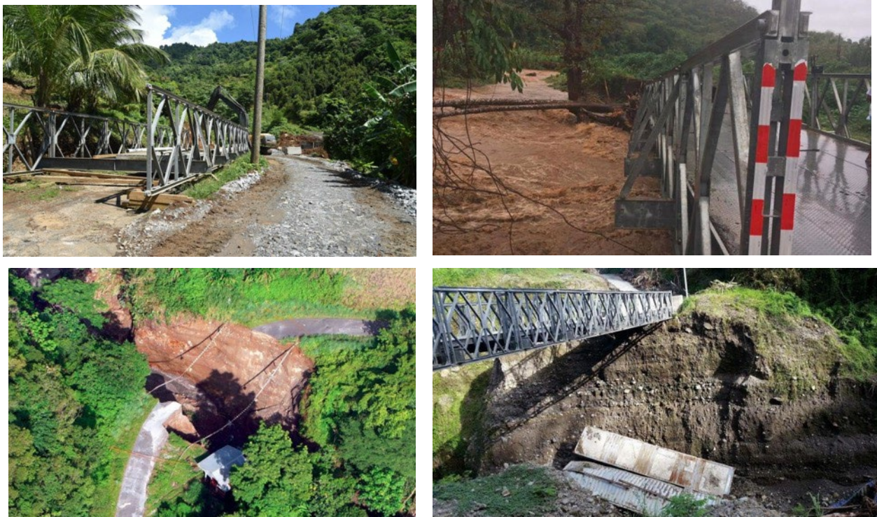
Figure 37: Showing the importance of Bailey bridges for maintaining accessibility in mountain Caribbean environments affected by extreme rainfall events. The lower images are of Boetica in Dominica, where a deep ravine was formed during a tropical storm that was crossed by a Bailey bridge.
